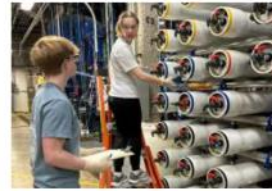
Kaden and Claire inspecting the Reverse Osmosis filtration system
